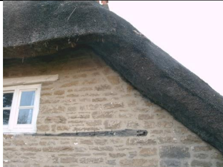
Original Wall Plate
